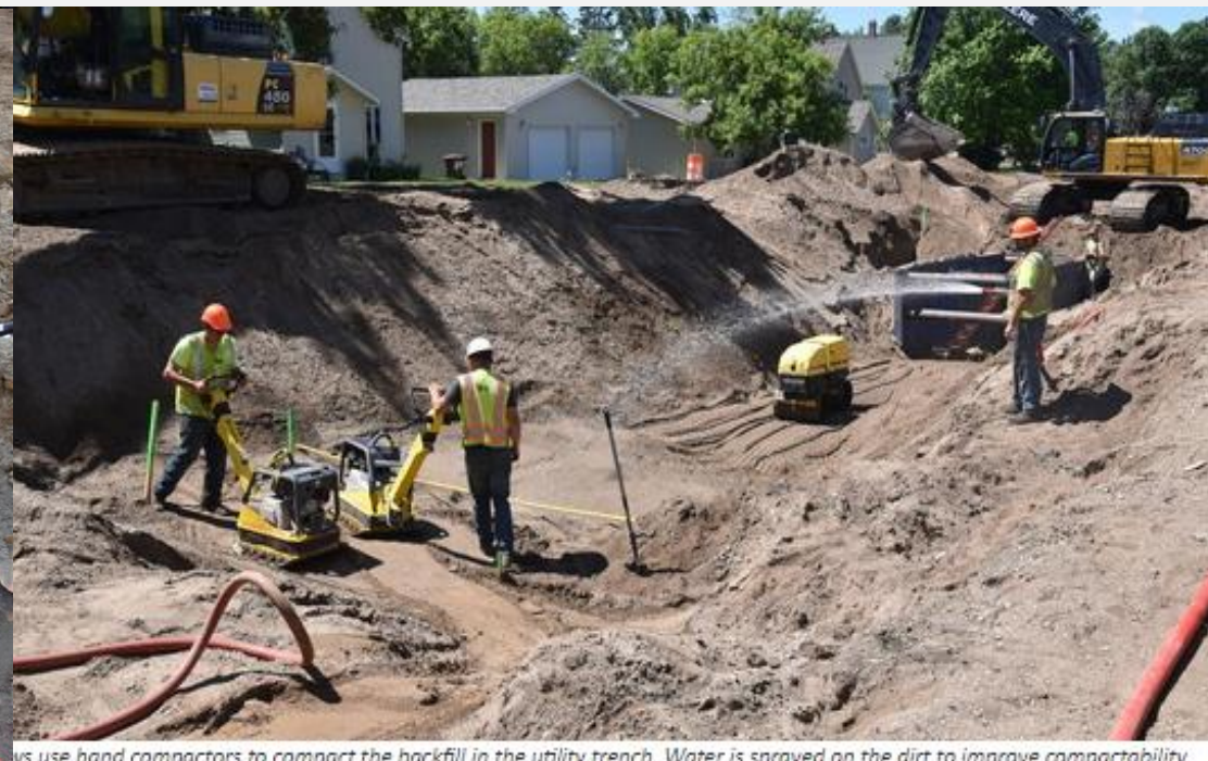
Workers use hand compactors to compact the backfill in the utility trench. Water is sprayed on the dirt to improve compactability.
